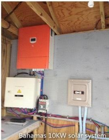
Bahamas 10KW solar system
