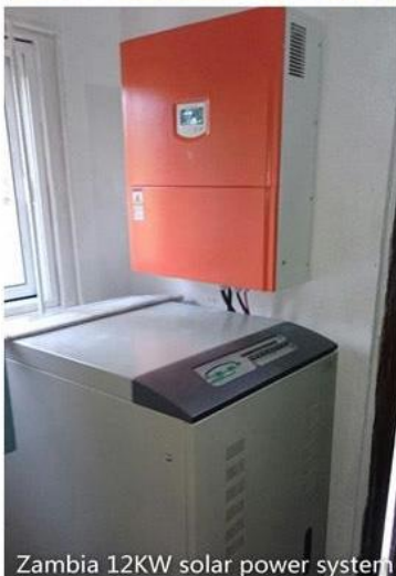
Zambia 12KW solar power system
